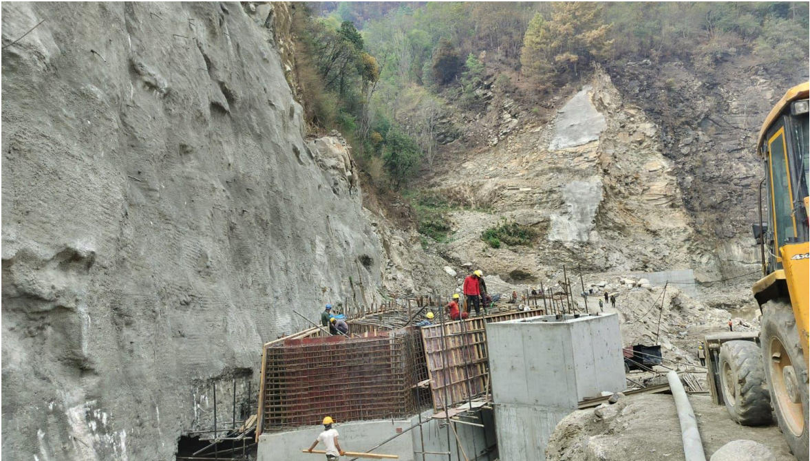
Secondary gravel trap
