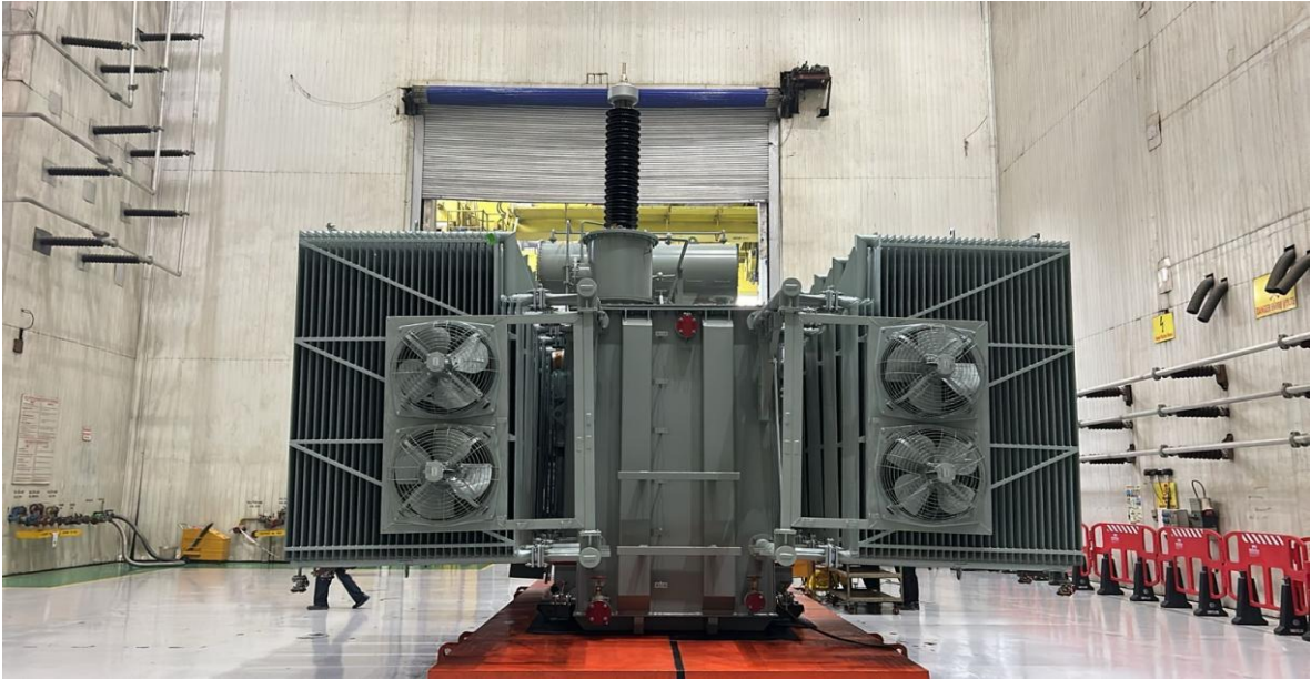
Power Transformer at Test Bench
