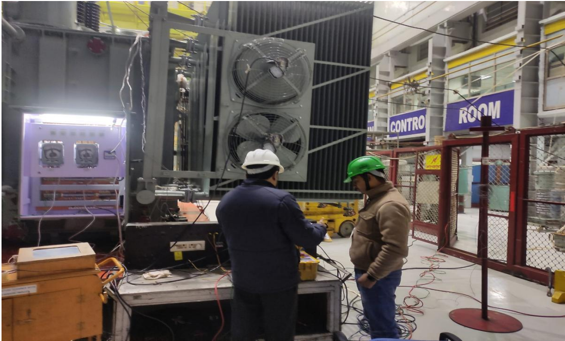
Measurement of Fan Loss in Power Transformer
